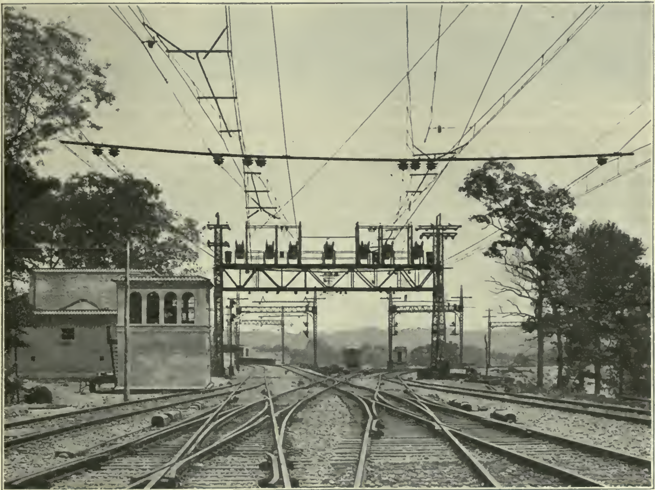
FIG. 523. SWITCHING STATION ON ANCHOR BRIDGE. 11,000-Volt Single-Phase Electrification, New York, Westchester & Boston Railway.
